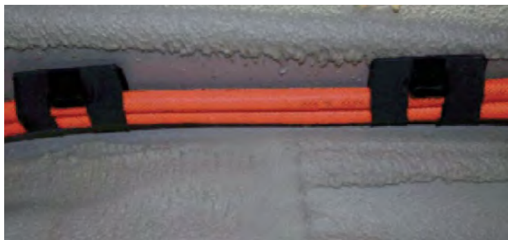
High-voltage cables can be identified by the orange-coloured insulation or coating.
