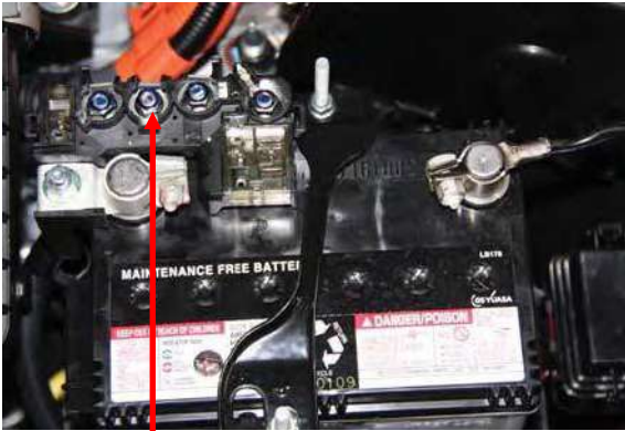
DC to DC Converter Cable Connection
