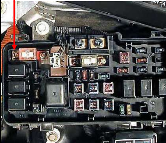
Main Fuse Screws
