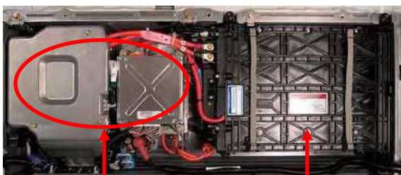
Other High-Voltage Components
