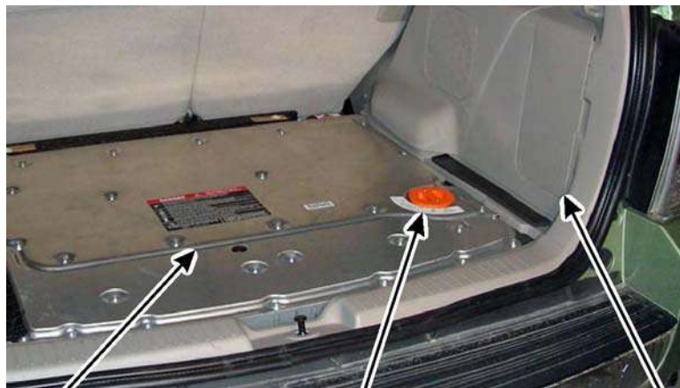
High-Voltage Battery Pack
